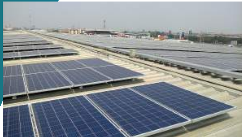
Being Subcontractor in installation labor for 999kW at Big C super Center Ayutthaya.
